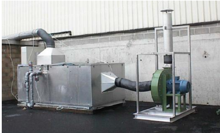
Picture 2 – SORBICAT pilot plant
