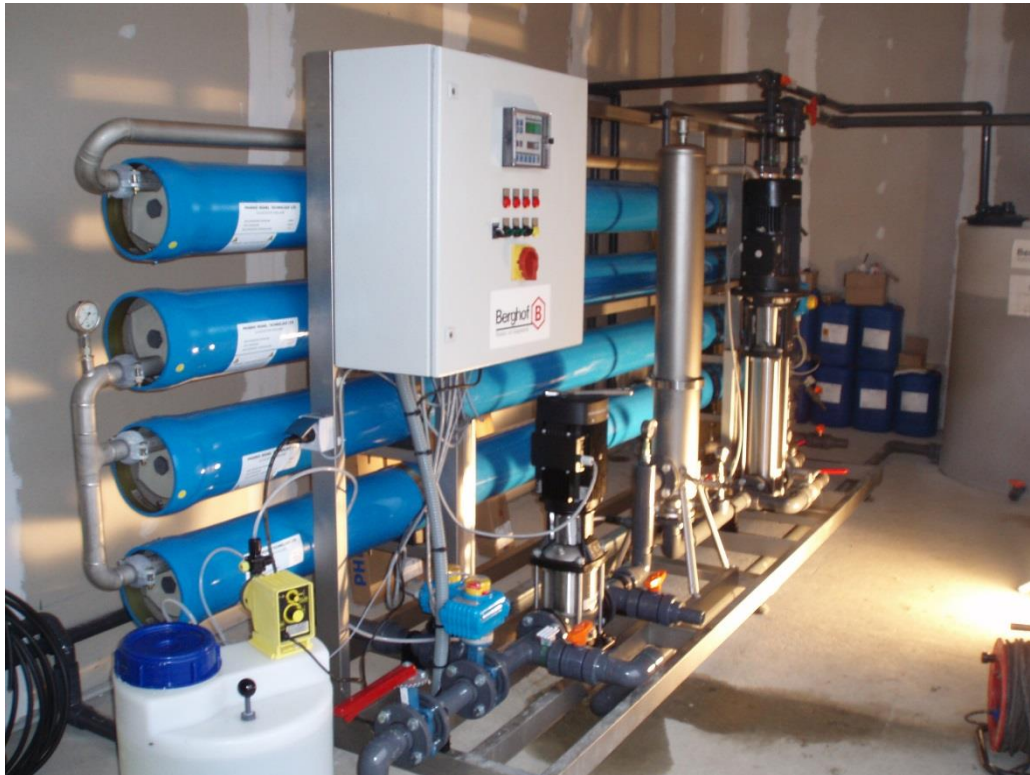
Picture: 1: Nanofiltration plant installed in France
