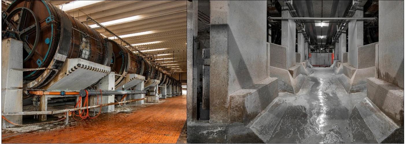
Figure 3: Beamhouse drums (left) and unloading channels (right)
