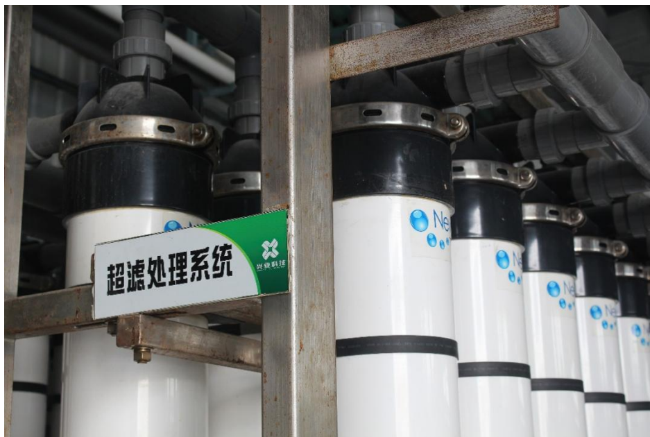
Figure 4: Detail of the ultrafiltration equipment
